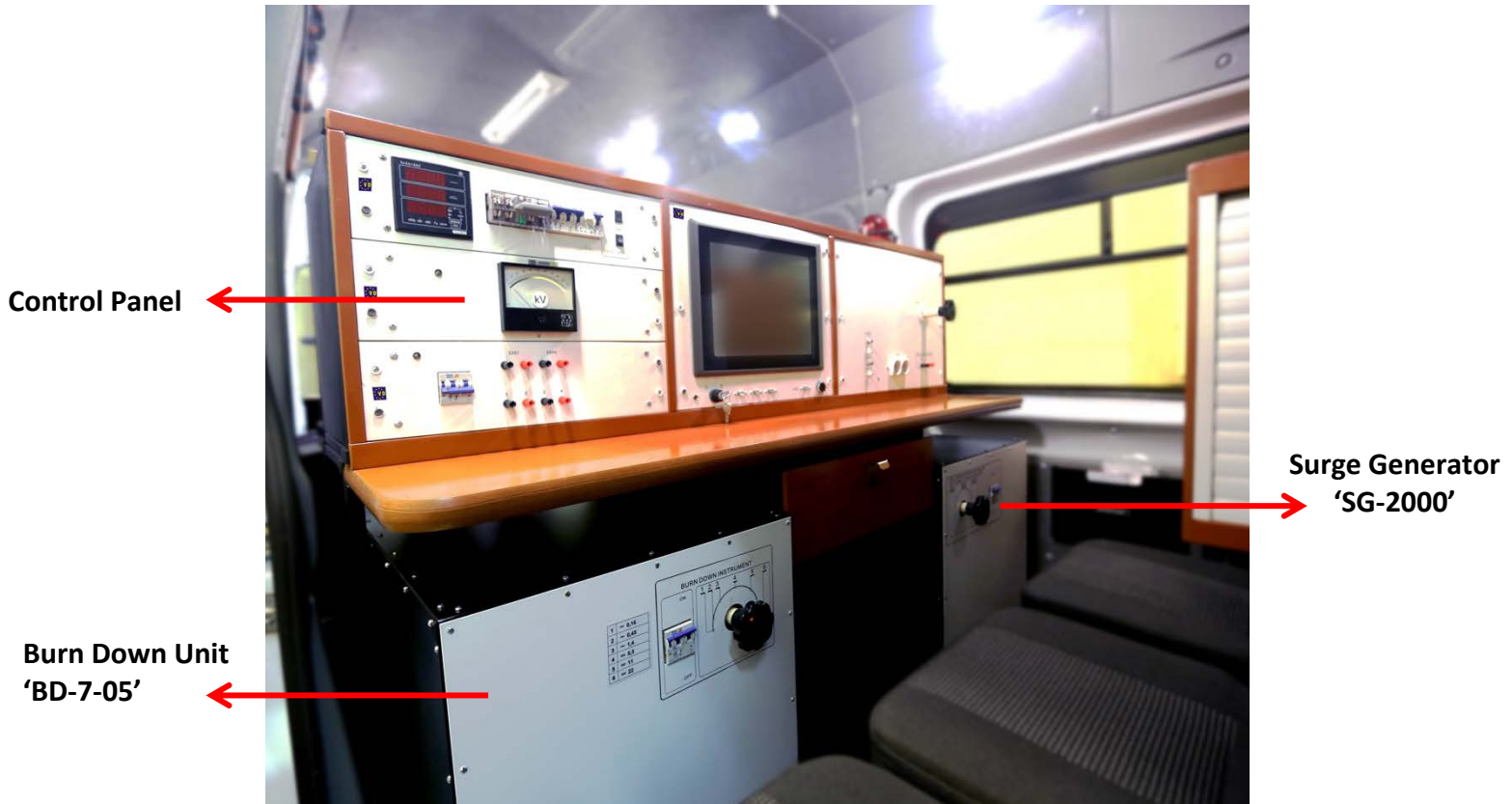
View of the Operators Area
