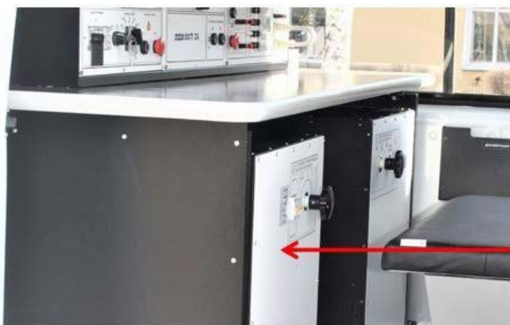
View of the Fault Burner 'BD-7-05'
