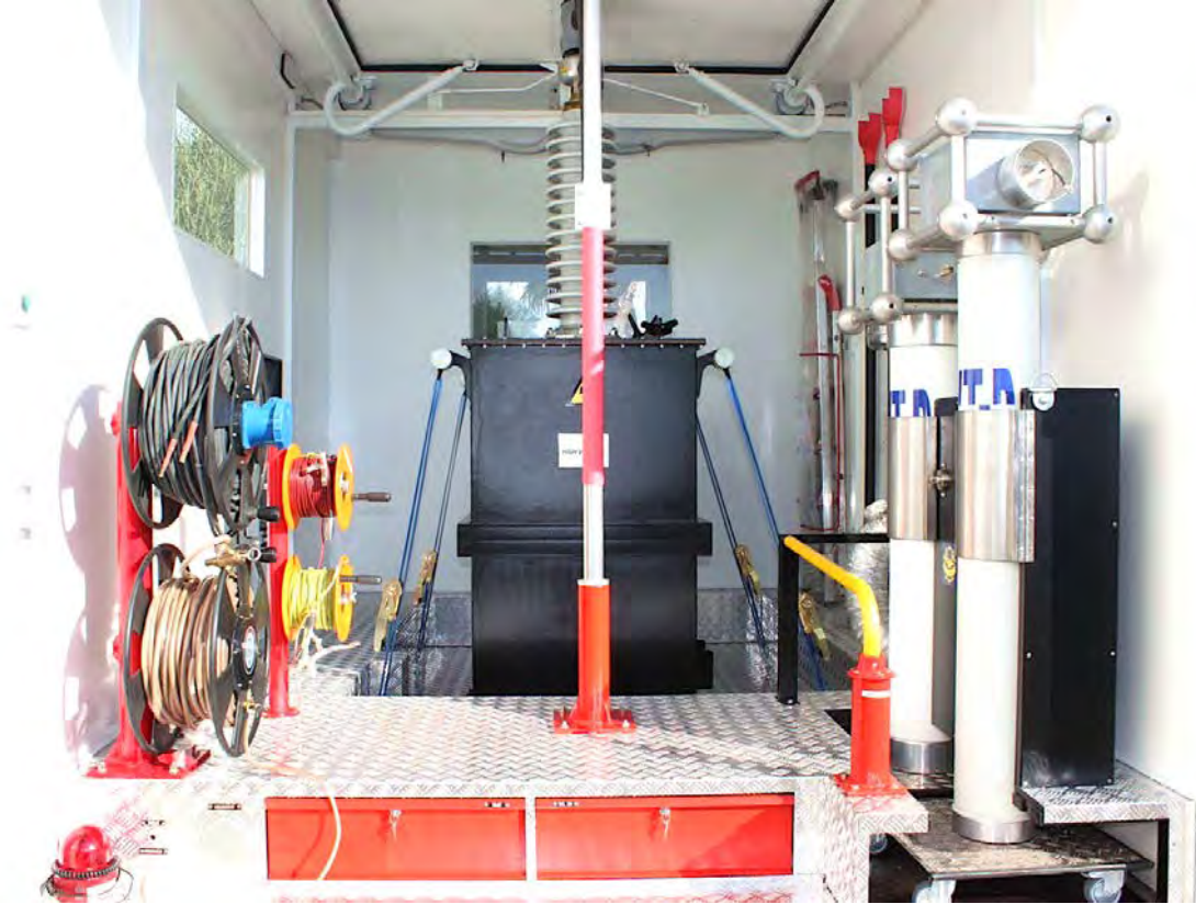
View of the High Voltage area *for reference only
