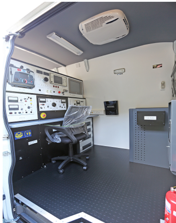
View of the Operator area
