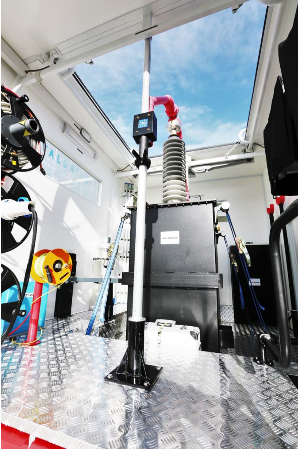
Fig. 5 View on the high voltage room
