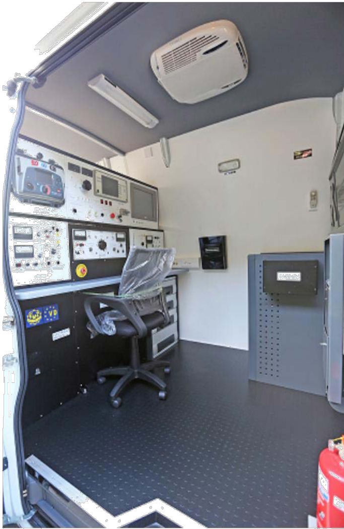
View of the Operator area
